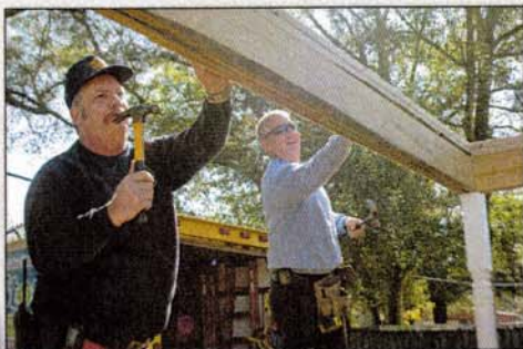
Fire Chief John Rebel (left) and Capt. Keith Vinson work on the front porch area of the Habitat home being built on Byrom Street. Vinson used to live at this very address some 23 years ago and now is helping to build the replacement home.
